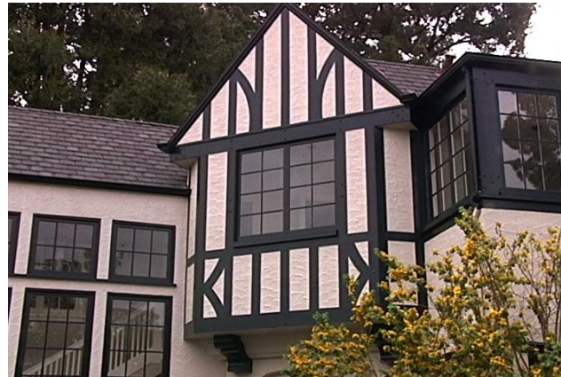
Windows at the addition to the left are consistent with the existing windows to the right.
